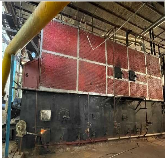
10t/h 气化锅炉
